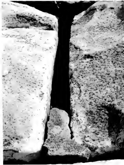
Figure 17: Loose and missing mortar from a joint in the rock mound base
